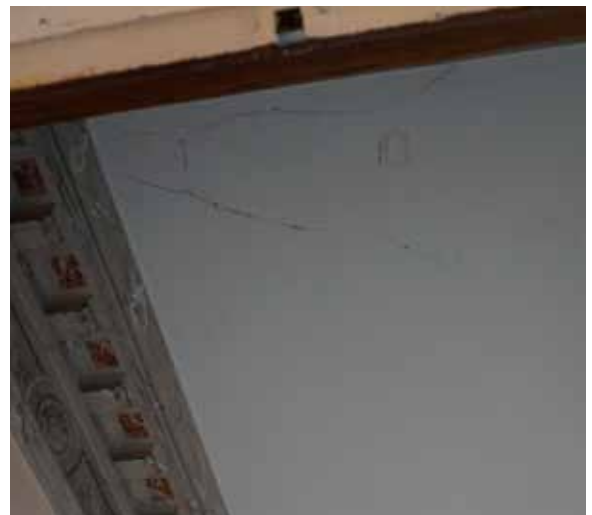
Sprickor i taket.
